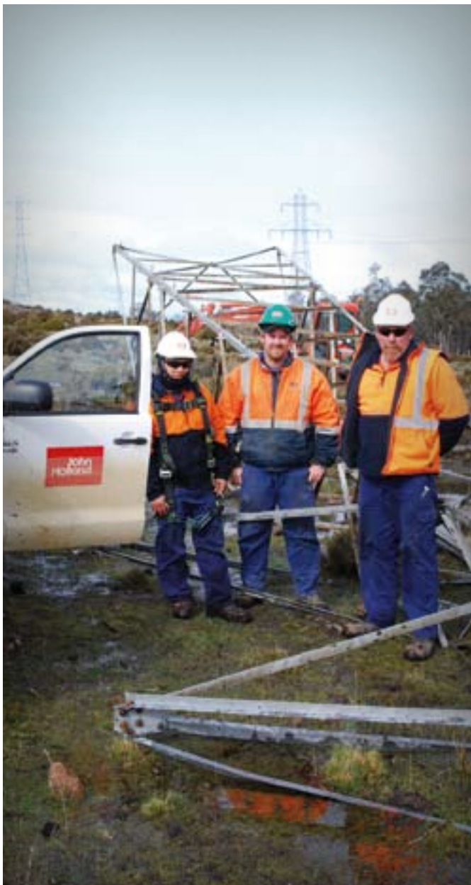
(from left) John Holland's Amado Fajol, Clint Wilkinson and Chris Baldock are part of a team that is dismantling Transend's old Waddamana–Bridgewater 110 kV transmission line. The old line is being removed to make way for a new Waddamana–Lindisfarne 220 kV transmission line
