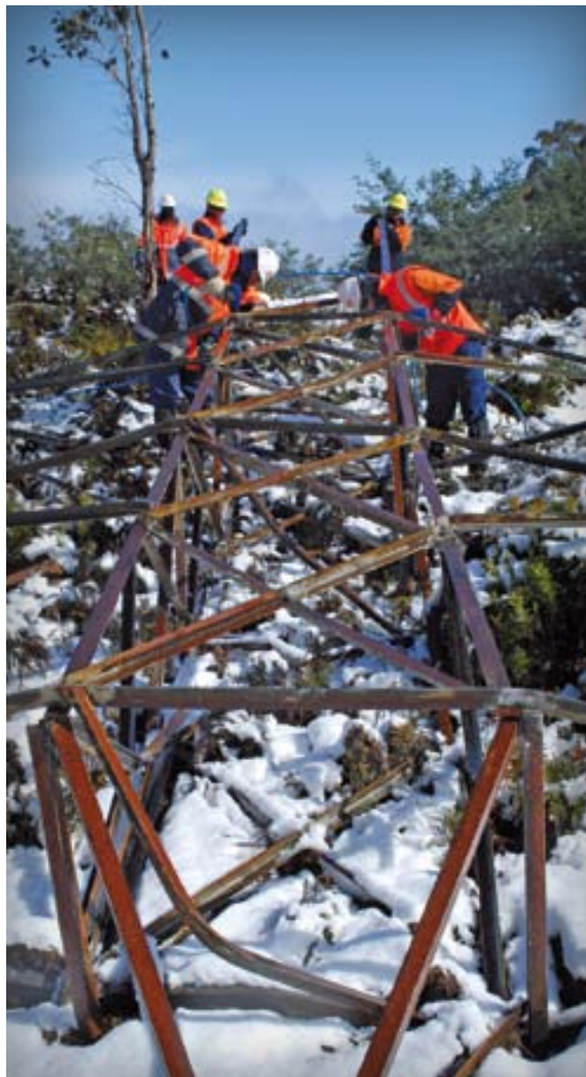
A John Holland crew dismantles a tower on the old Waddamana–Bridgewater 110 kV transmission line
