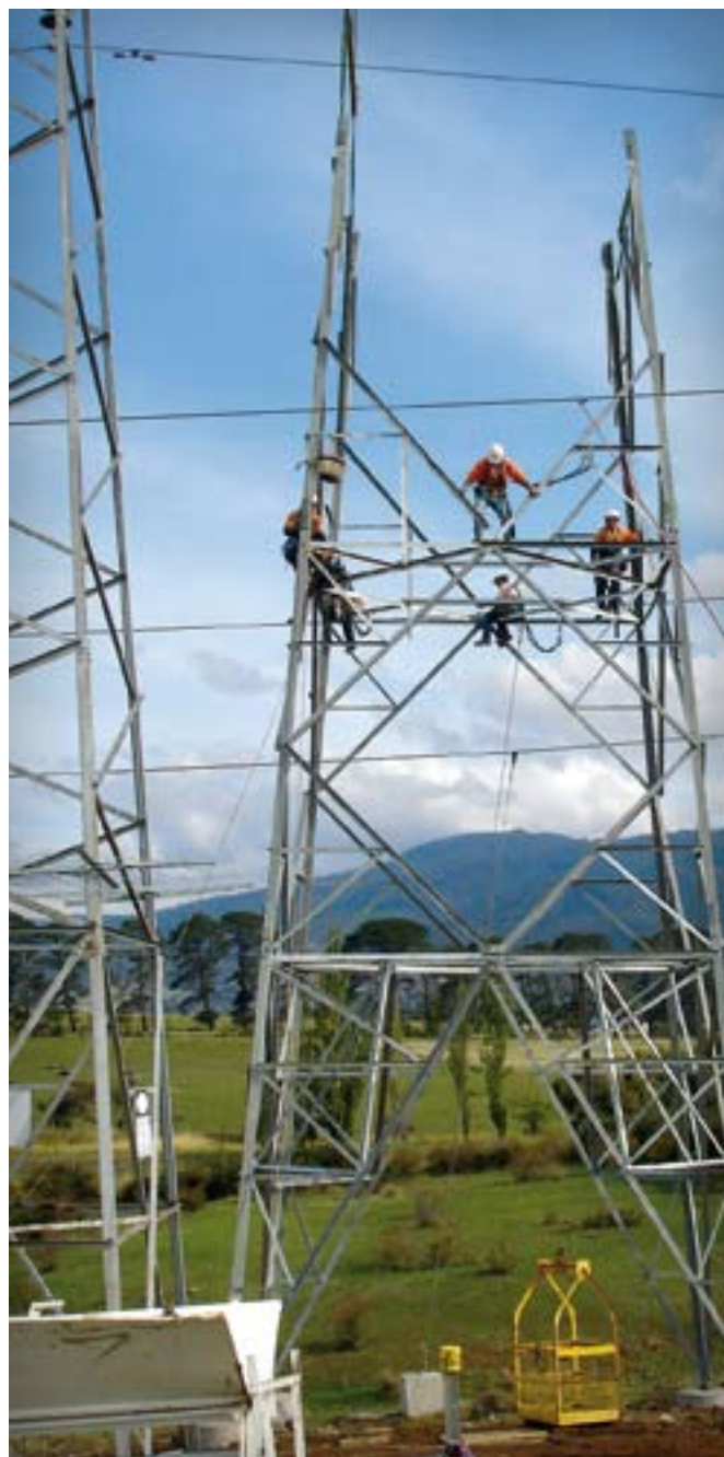
A Transfield Services crew constructs a new tower on the Waddamana–Bridgewater 110 kV transmission line
