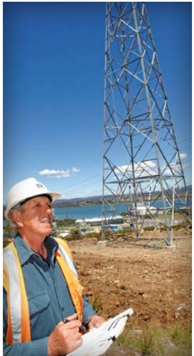
Transend's Carl Hankey, works inspector, oversees construction work on the George Town–Tamar Valley Power Station 220 kV transmission line. The Tamar Valley Power Station, still under construction, is in the background
