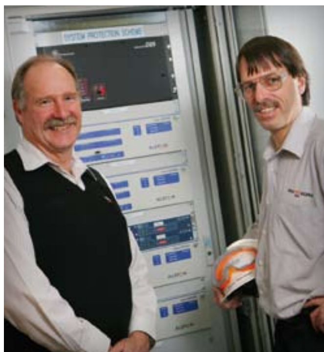
(from left) Transend's John Peter, metering/customer account manager, with Nyrstar Hobart's David Gaskell at Nyrstar's electricity substation. Nyrstar is one of Transend's major industrial customers
